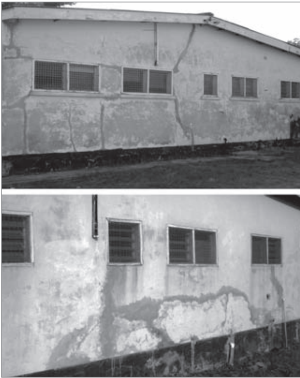
Figure 1: Patched cracks in a home located in Tema, Ghana; non-professional maintenance by occupants (photo: Laurence Amedzro).
